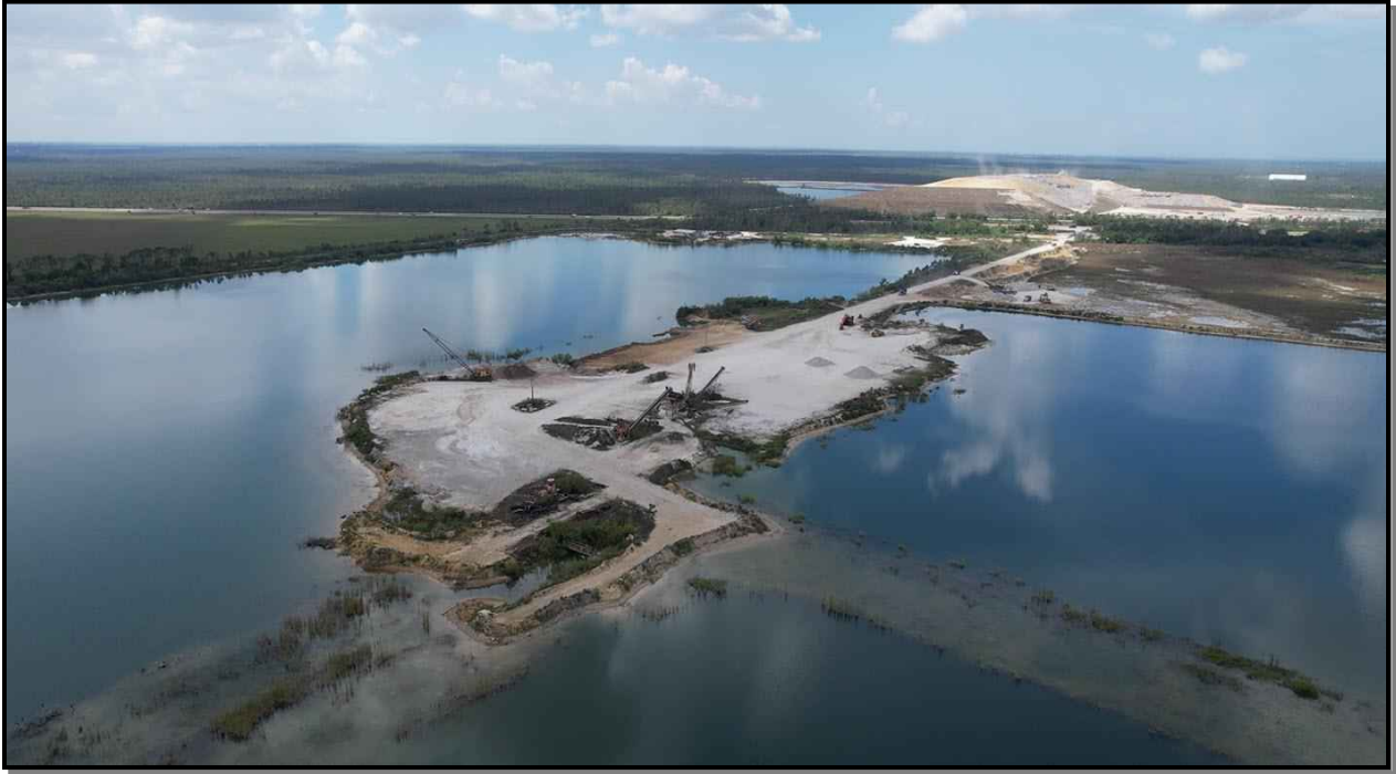
Looking southwest across the rock processing area with the County landfill in the distance
